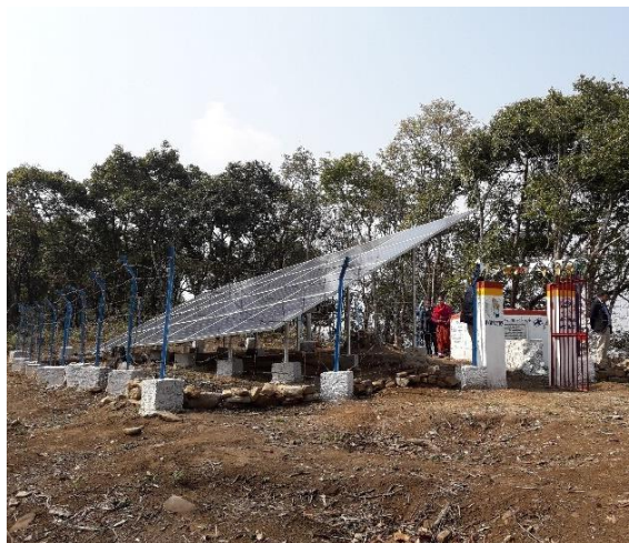
Photo: Solar panels for solar water pump in Balikot
